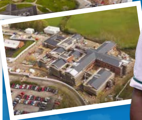
Great progress is being made on our three completely new buildings: the Carsington Unit and Kingfisher House in Derby and the Derwent Unit in Chesterfield
